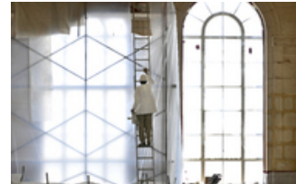
An employee of Lobar Inc. of Dillsburg works on renovating trim around the front windows at the Lancaster train station interior. (Dan Marschka)
