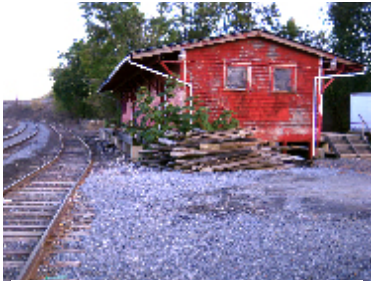
Plans to move a wood-framed freight station on South Wilson Avenue for overflow parking at the Elizabethtown Train Station are underway. (Chad Umble)
